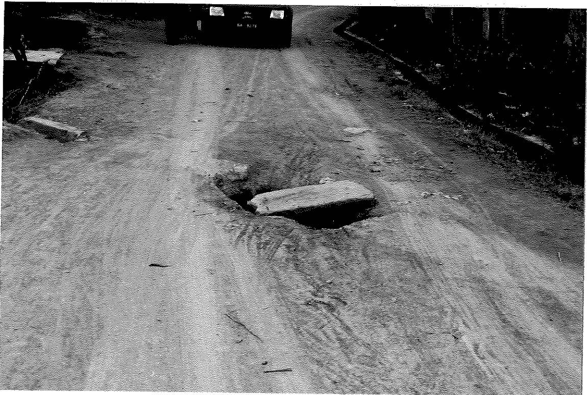
Photograph - 2: Dheri-Mallhu Road (Godo Link) showing damaged drain crossing the road
