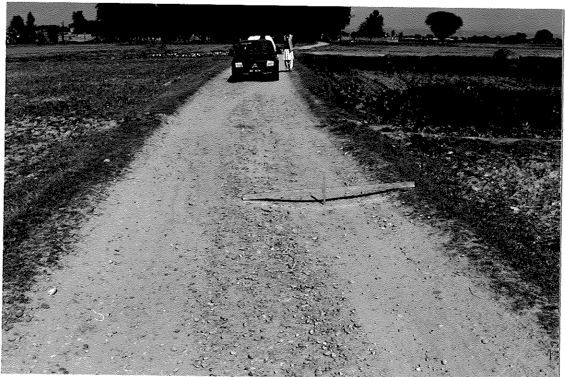
Photograph - 20: Sheikh Qureshian Road showing gravel loss and rutting of surface
