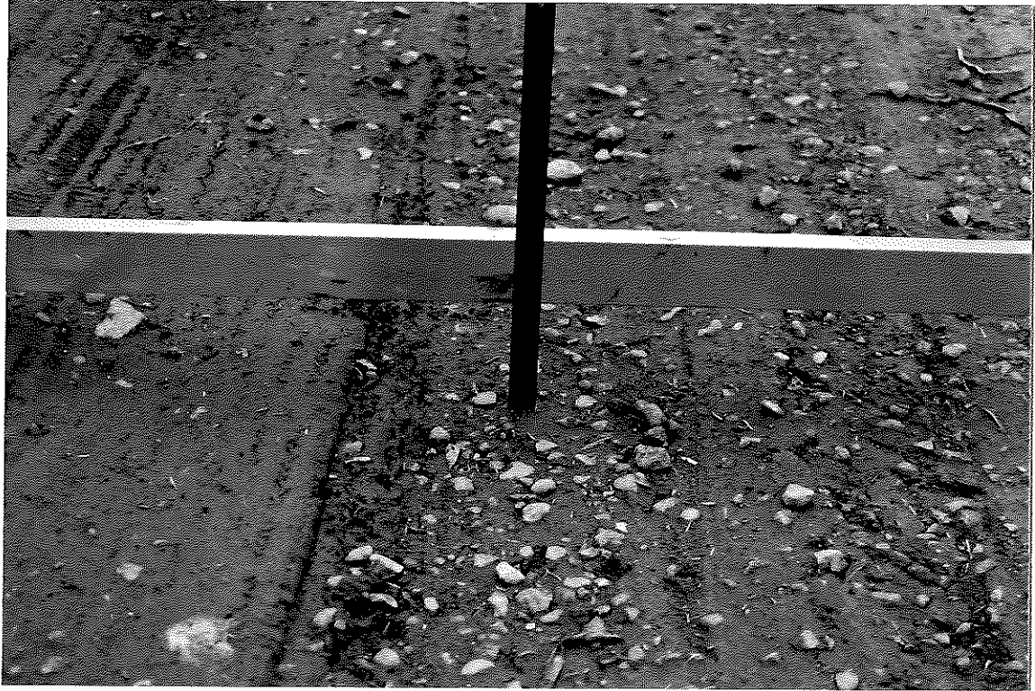
Photograph - 15: Humak-Jawa Road showing 4" depression in the surface
