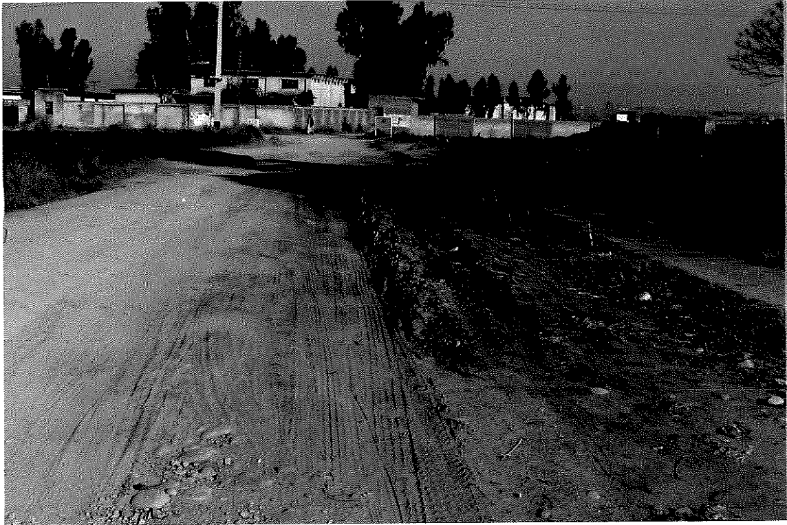
Photograph - 13: Humak-Jawa Road close view showing gravel loss
