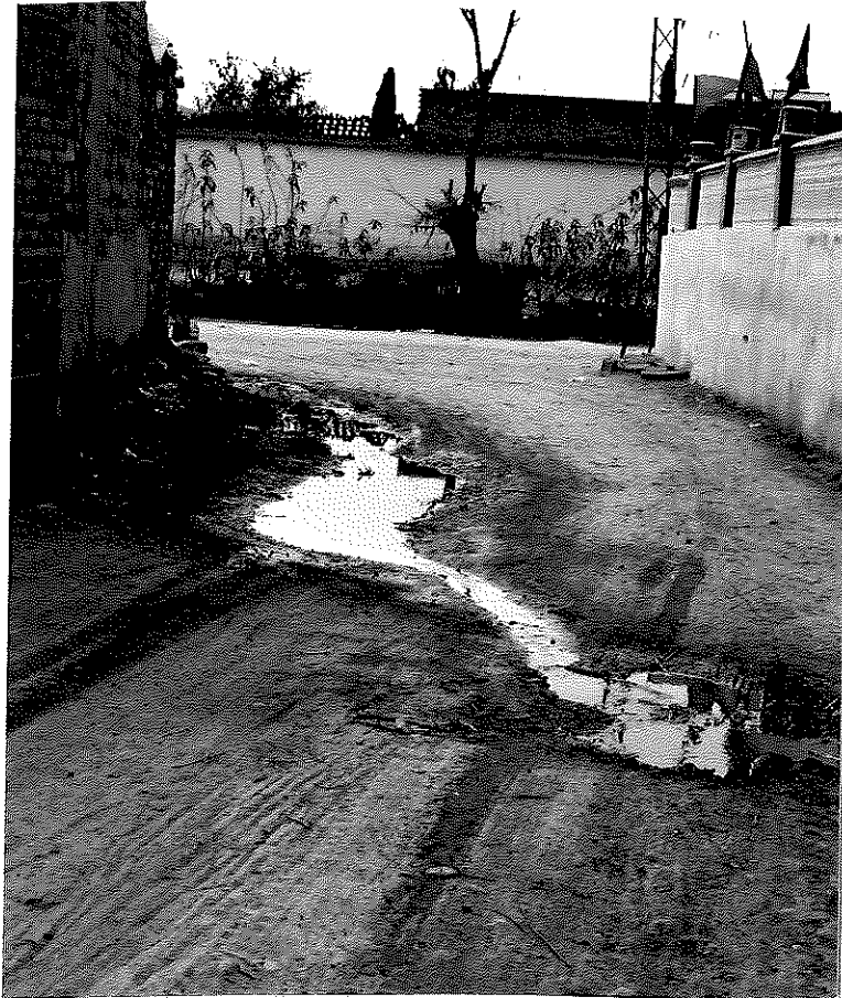
Photograph - 1: Dheri-Mallhu Road (Godo Link) showing open drain crossing road.
