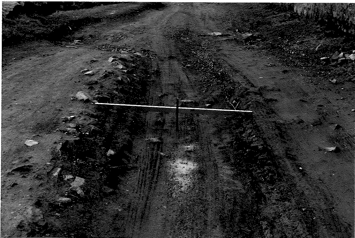
Photograph - 8: Dorro Village Road showing 9" deep depression corrugation/rutting
