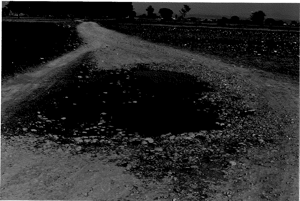
Photograph - 18: Sheikh Qureshian Road showing water ponding
