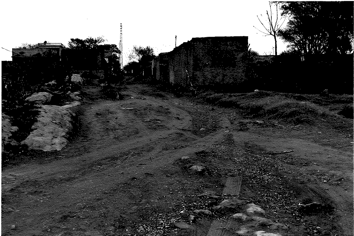
Photograph - 7: Dorro village Road showing damaged low cost road near village "Parrian"
