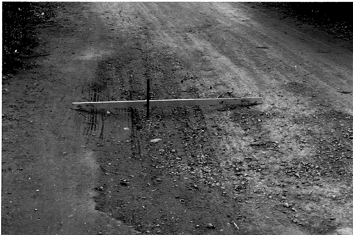
Photograph - 4: Dheri-Mallhu Road (Godo Link) showing big depression with gravel loss
