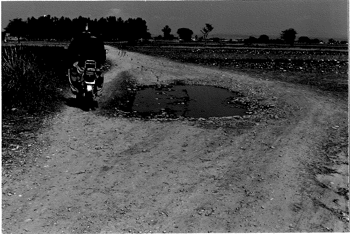
Photograph - 19: Sheikh Qureshian Road another view of water ponding
